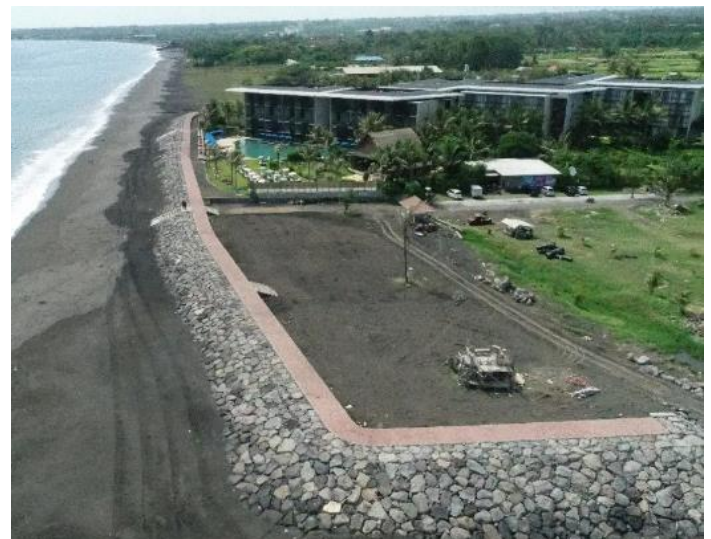
Figure 3. Construction of roads and barriers between villas and beaches to support safety and comfort for tourists in Klungkung Regency.
